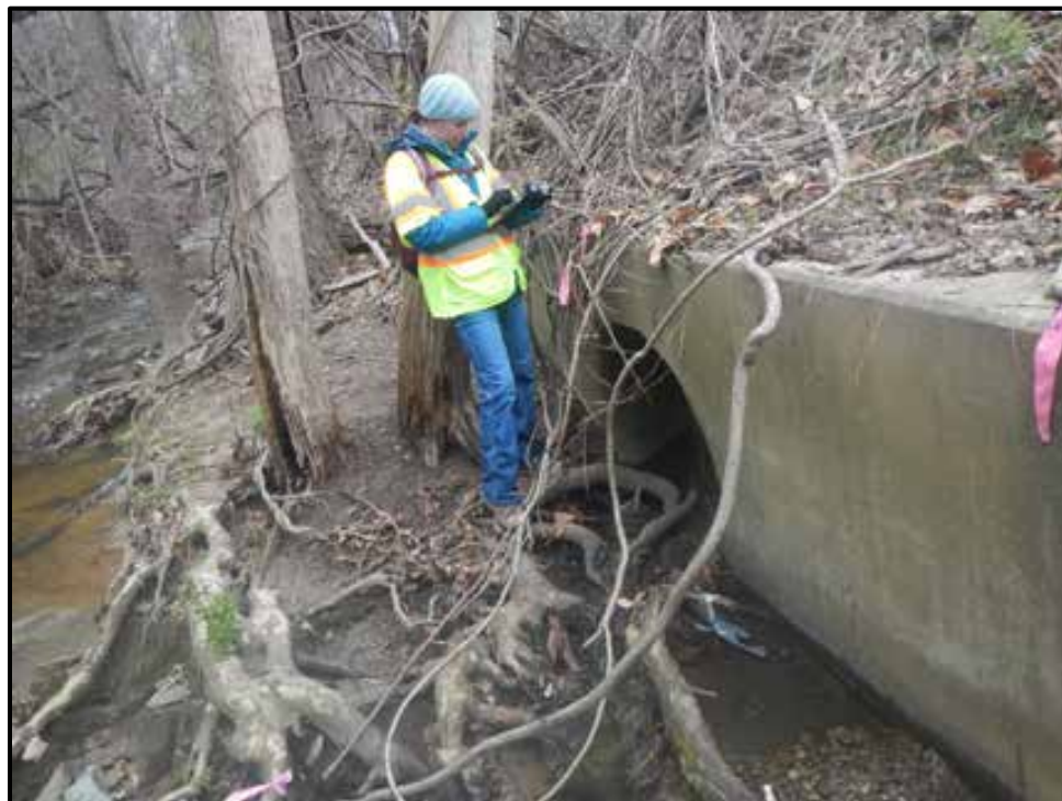
Waterway 21I – Perennial
